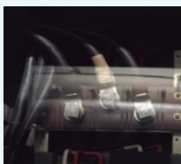
An abnormal exothermic of wiring
